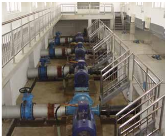
Conveying Pump House in Tianjian, PRC
