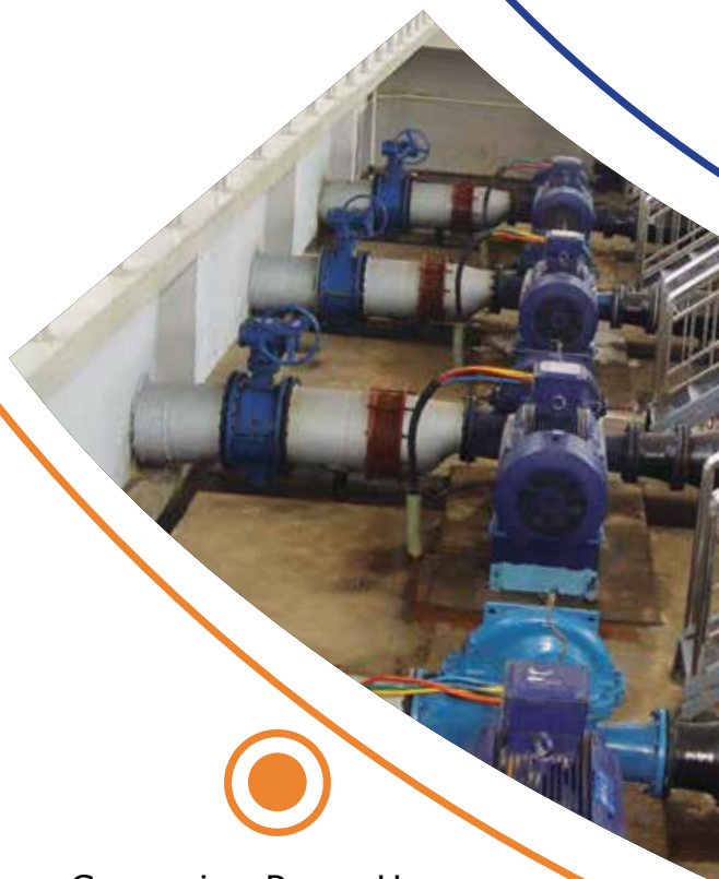
Conveying Pump House in Tianjian, PRC
