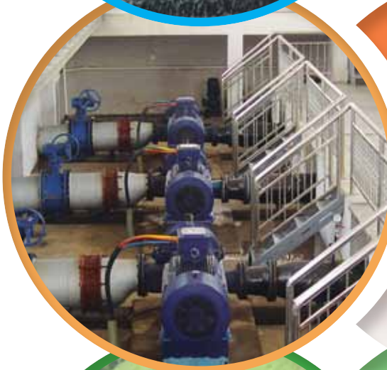
Tianjian, PRC Conveying Pump House
